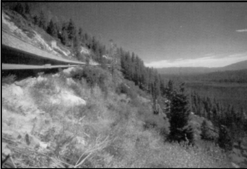
Typical area along highway that is subject to rock slides.
