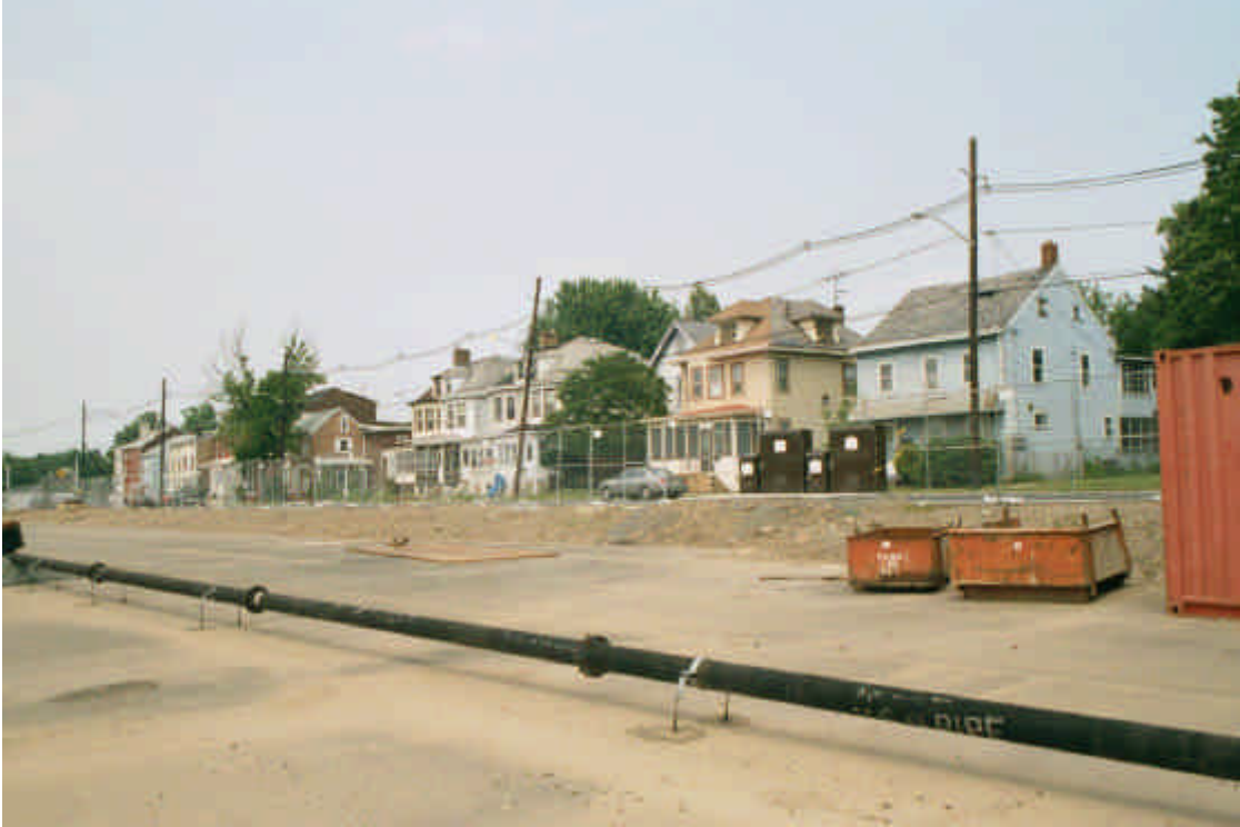
E.11 Roof deck of tunnel that will become park looking toward historic homes along Lamberton Road.
