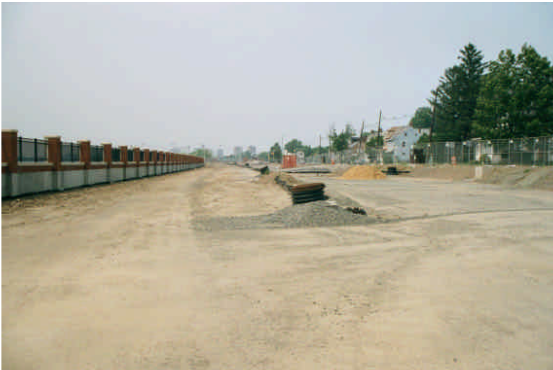
E.10 Roof deck of tunnel that will become West Riverwalk Park. Fill will be added to brick line on wall on left side of photo.
