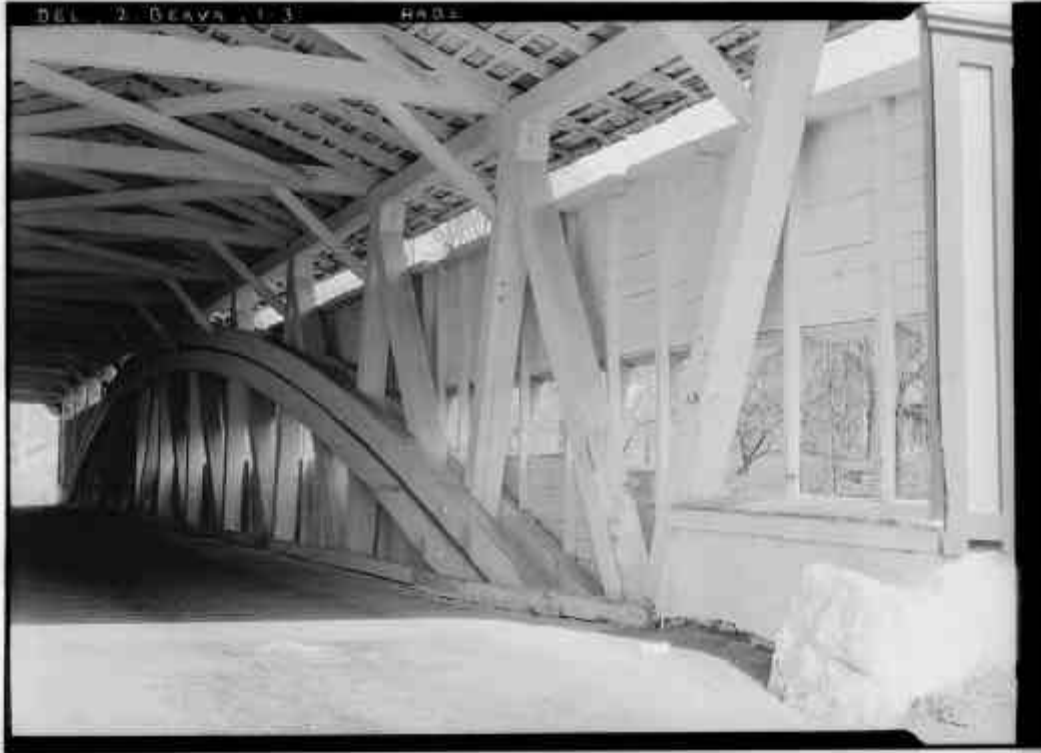
B.11 HABS photo of Smiths Bridge showing interior of 1839 covered bridge. Photo was taken in 1939.
