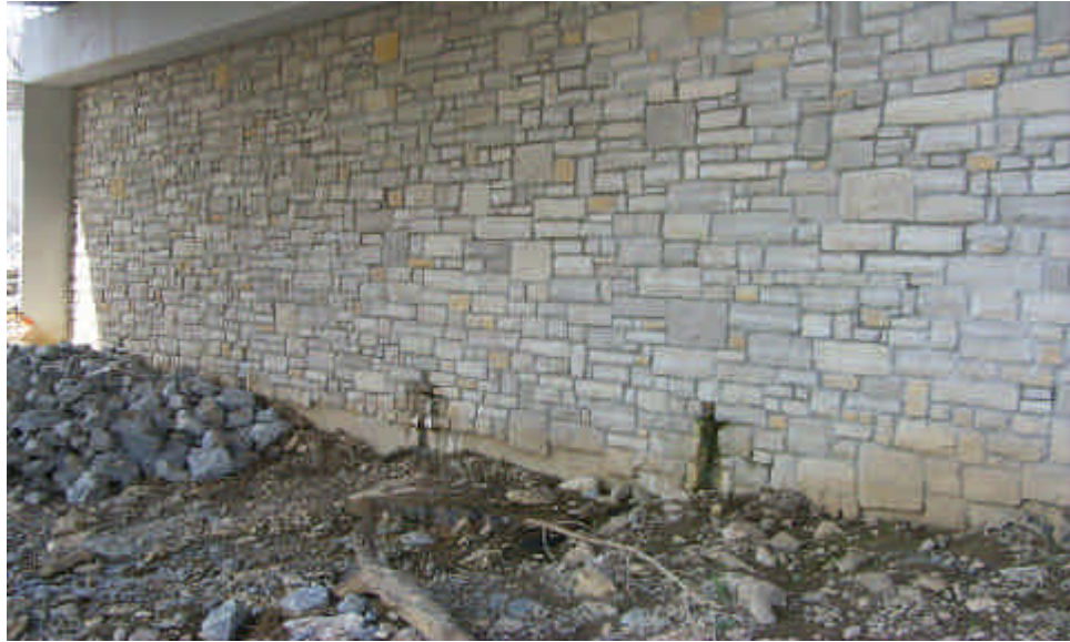
A stone facade to match the local indigenous stone outcrops was applied to the bridge structures near Paris
